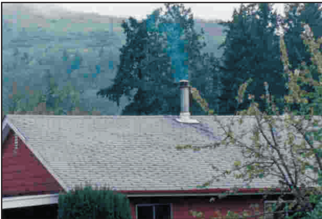
Chimney smoke should be negligible when a woodstove/fireplace is being properly used.
